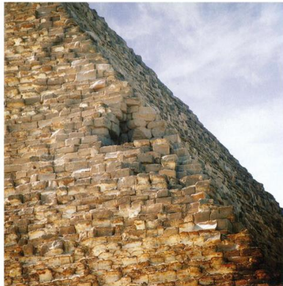
Figure 8: Notch on the northeast corner
